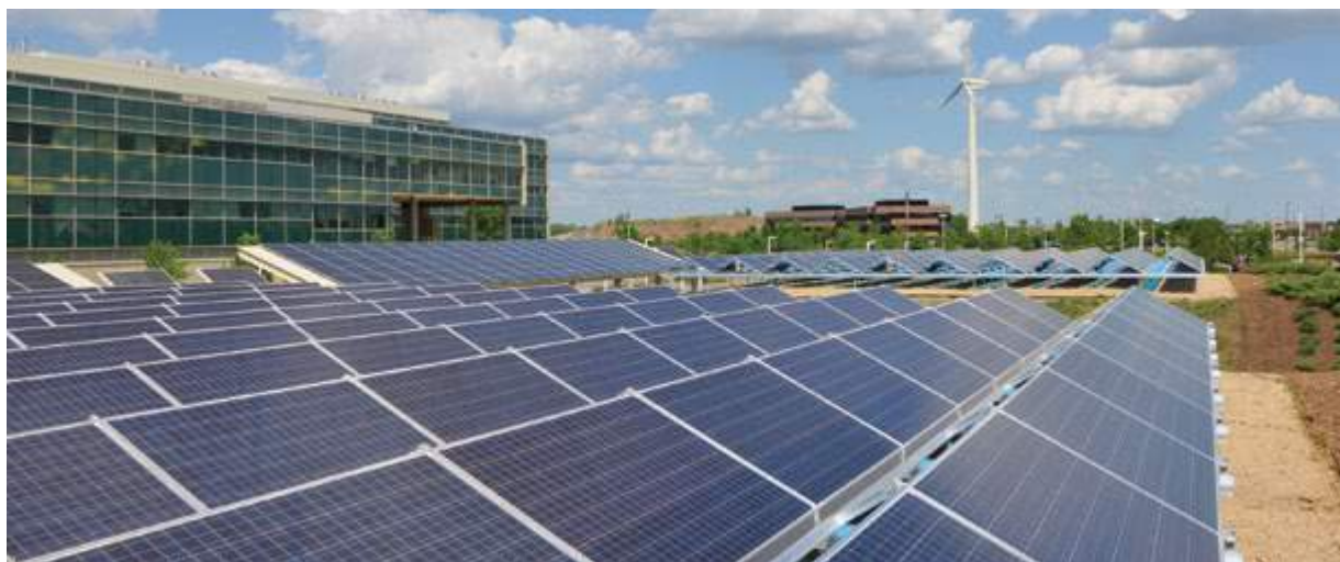
The cooperative solar installations will employ solar technology from Minnesota companies tenKsolar and Silicon Energy. Energy Concepts installs and commissions the projects.
